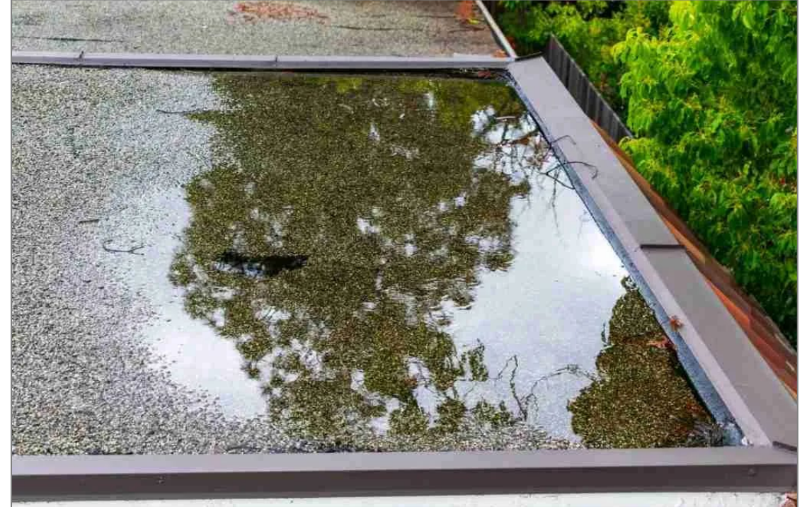
deflection of flat roof leading to water accumulations
