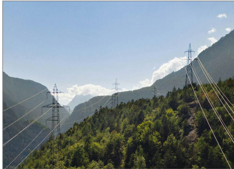
Electricity pylon Swissgrid
